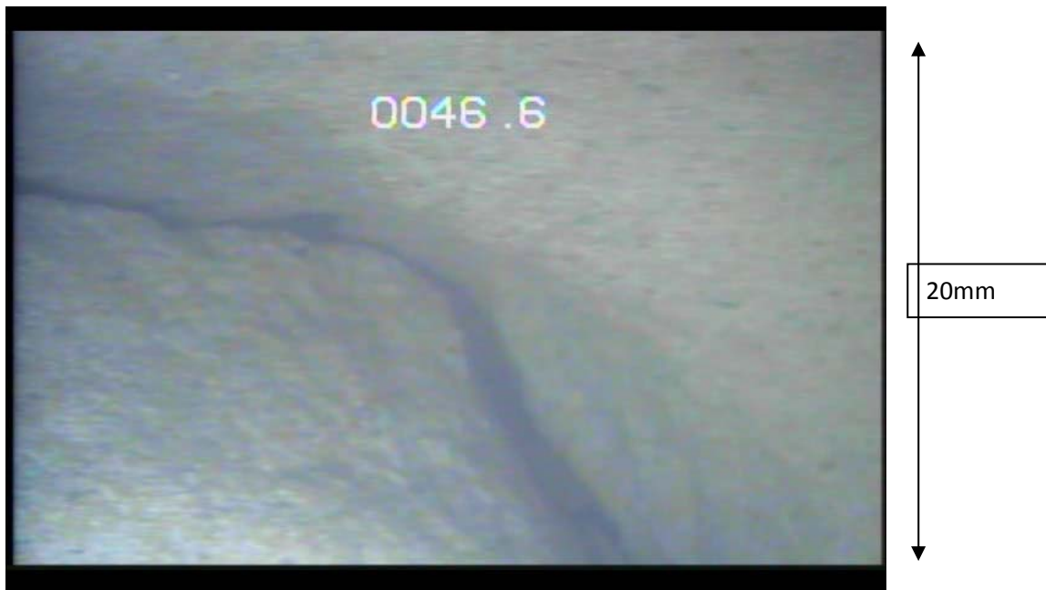
Photo 4: DH Qu10-17 14m depth. Constrained zone. Pre-existing fracture encountered large inflow of water during drilling.
