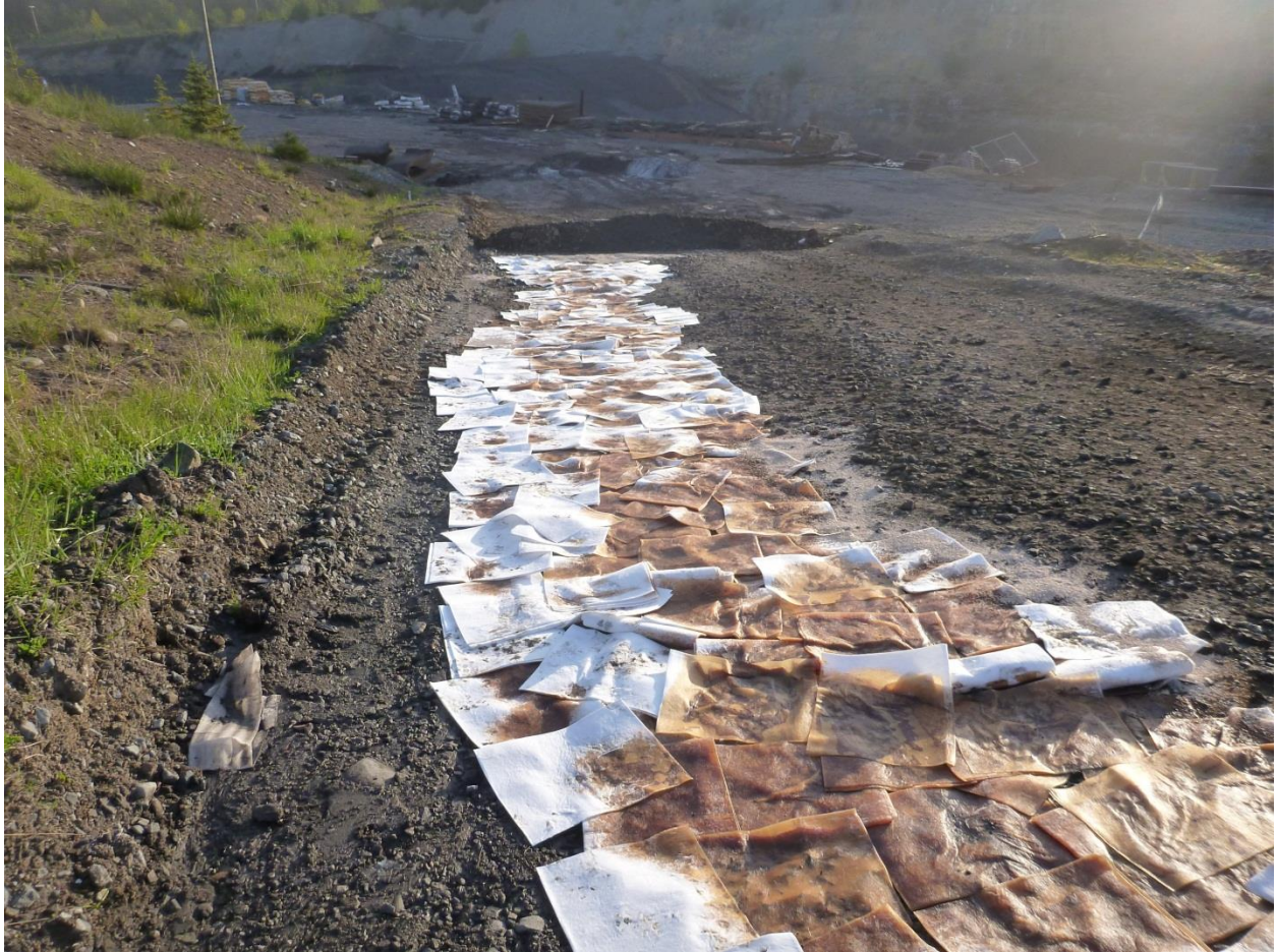
Plate 2. – Location of the fluid spill downhill from the damaged machine, with a containment berm constructed near the downhill base of the grade.
