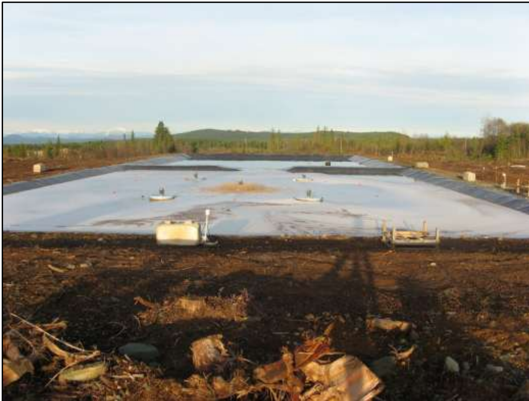
Photograph 16: Aerobic Cell with Aerator and Mixers (settling pond in the background)
