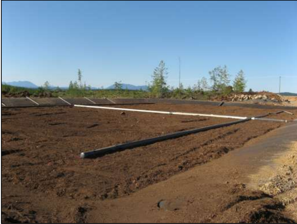
Photograph 15: Substrate (mixture of wood chips and iron) and Upper Piping in the Sulphide Polish Cell
