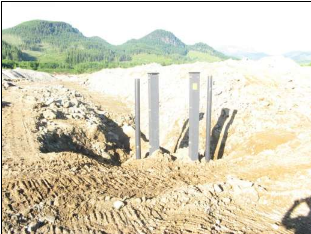
Photograph 8: Installation of the Water-Level-Controllers in the BCR Cell
